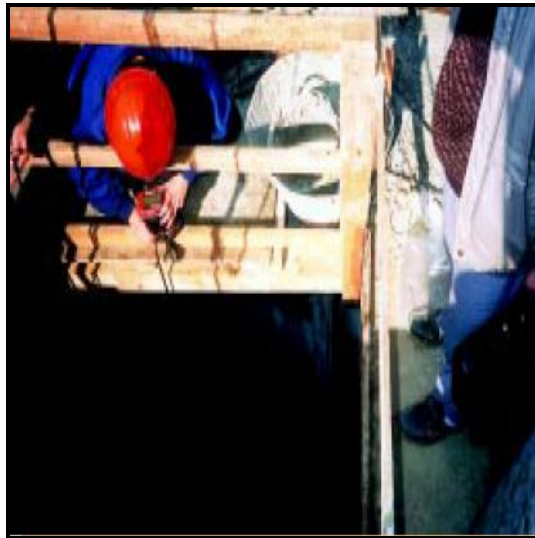
Figure 4. 8: Picture showing impeding external edge lighting connection
