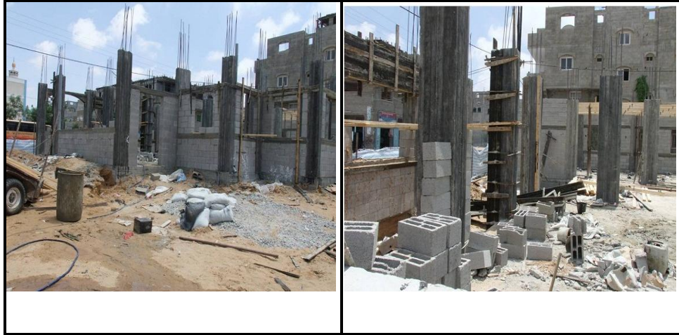
Figure 4. 14: Two pictures showing untidy job sites
